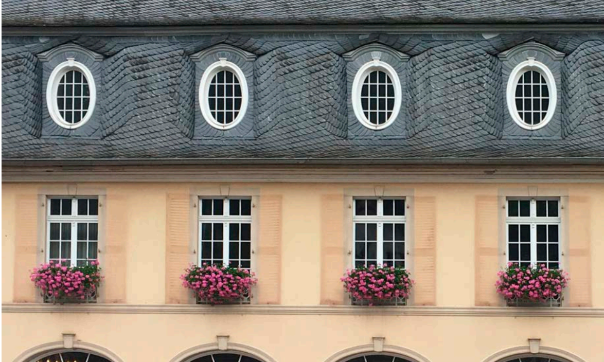
Facade with clearly visible colour changes in the areas of dismantled shutters.
