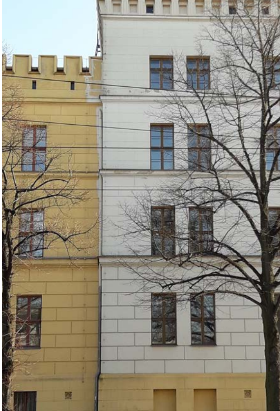
District recruiting office in Potsdam (left), painted in 1992 with KEIM silicate paint (colour shade 9071). Right: This part was coated with an organically pigmented paint from a competitor in the same colour shade, but clearly shows a colour change!
